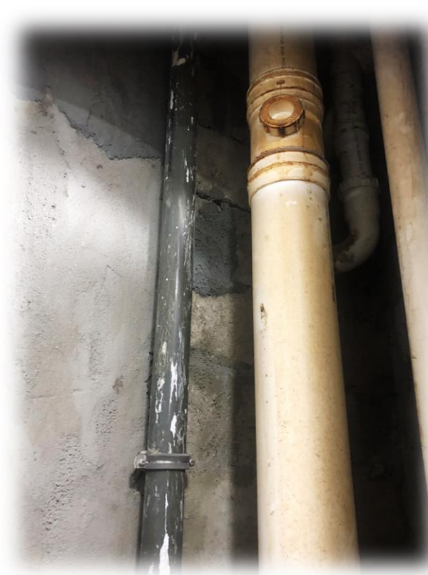
Internal pipe duct accessible from common parts
